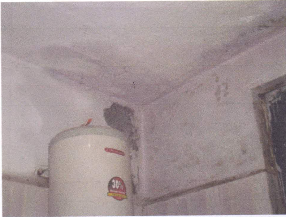
Damp patches in the bathroom wall.
