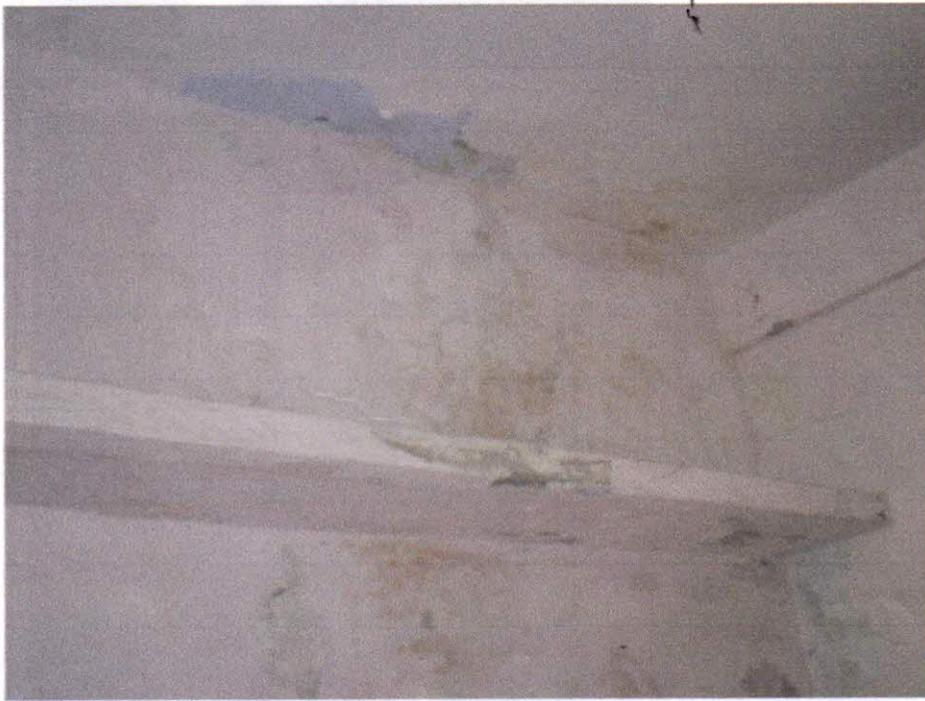
Stained surface of the wall due to the moisture content in the wall.
