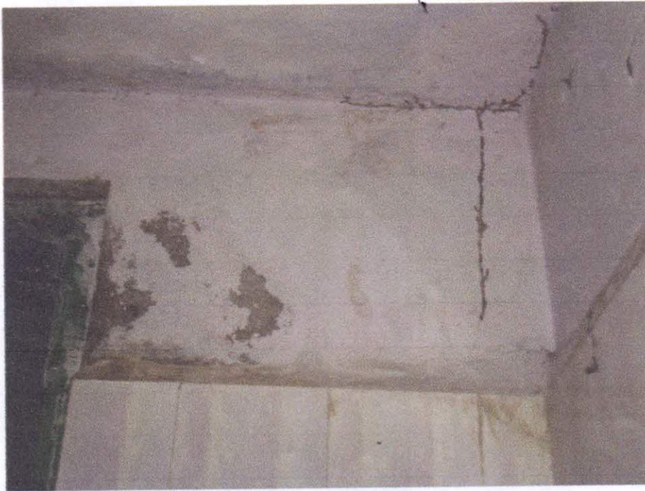
Moist surfaces and chipping off plaster in the toilet.
